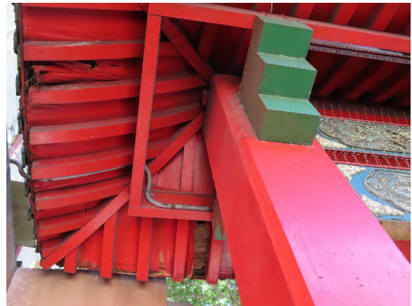
Figure 4.48 Deteriorated timber rafter and damaged plywood soffit.
