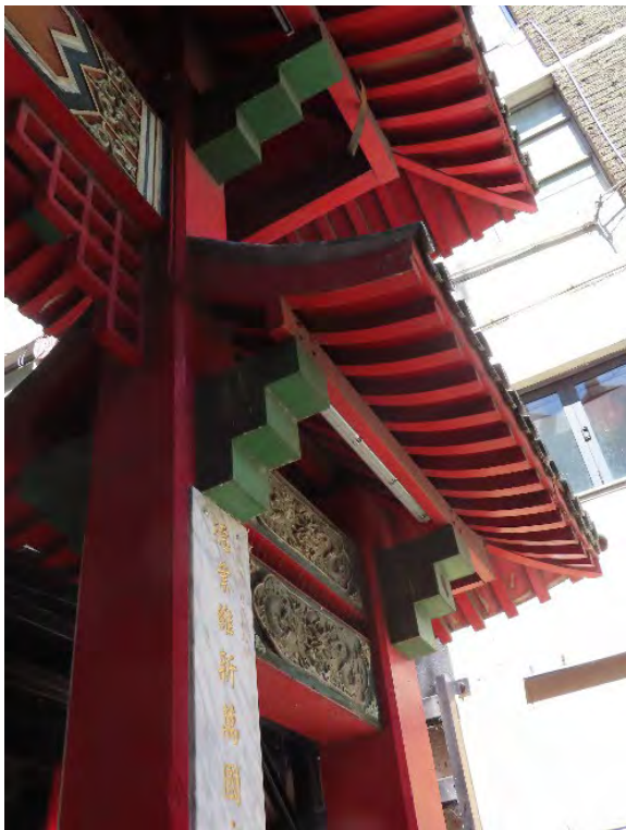
Figure 4.6 Underside of the curved timber rafters and stepped brackets of the west gateway, showing the lower and upper roof of the north elevation.
